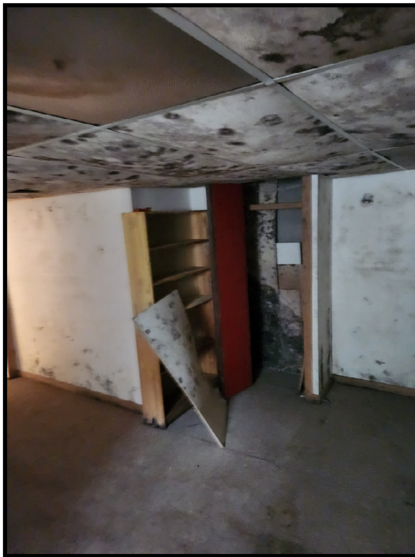
Photograph 7: mouldy basement finishes, where present
