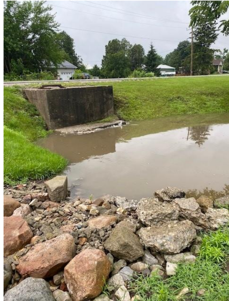
Image 11: Flooding within swale adjacent to 10990 Graham Road on July 29, 2023
